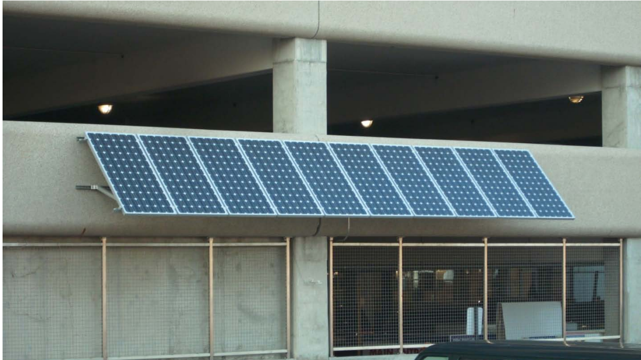
Figure 15: Photovoltaic (PV) Panels on Parking Structure
